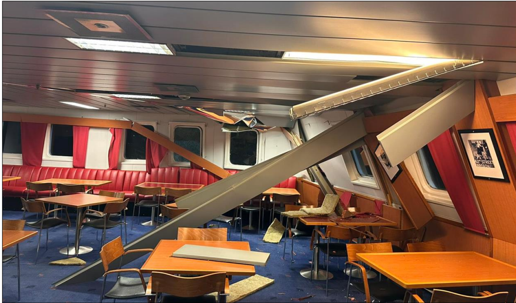
Fig. 7. Damaged Patria Seaways restaurant premises on deck no. 6 (photo provided by the Patria Seaways operator)
