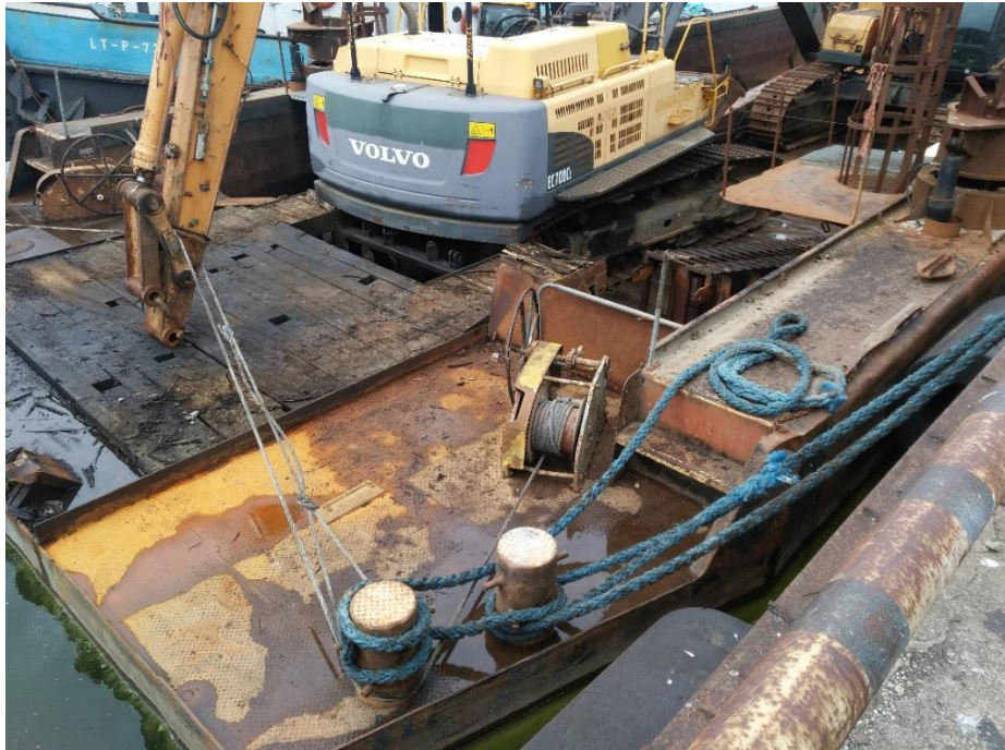
Photograph 4. Fastened arm of one of the excavators (Photograph taken by LTSA 3 inspectors)
