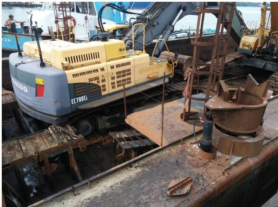
Photograph 5. Position of the excavators on the pontoon without fixing (Photograph taken by LTSA inspectors)
