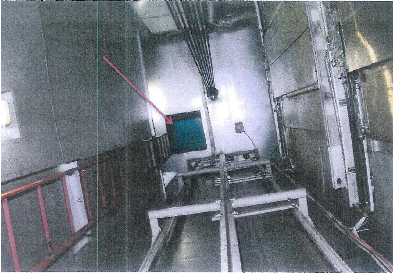
Figure 7. The equipment of emergency landing from the lift shaft.
