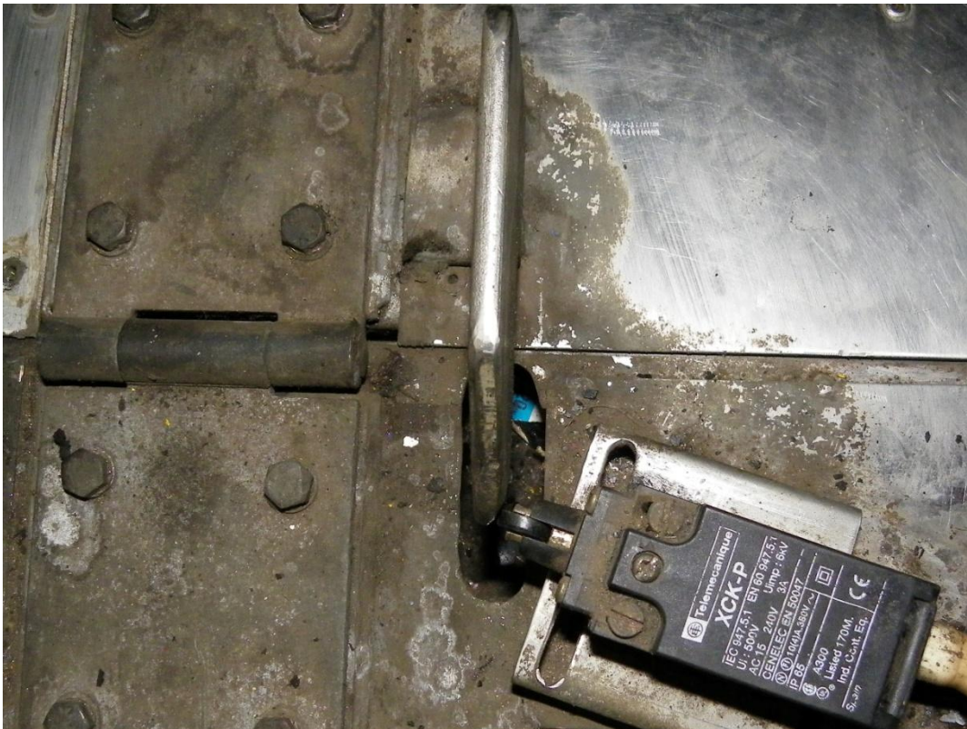
Figure 11. The switch of electric current of emergency hatchway of the lift when the cover is open.
