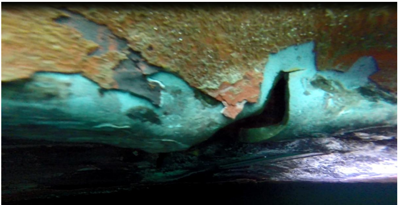
Figure 7. The hole in the hull resulting from the ship's running aground
